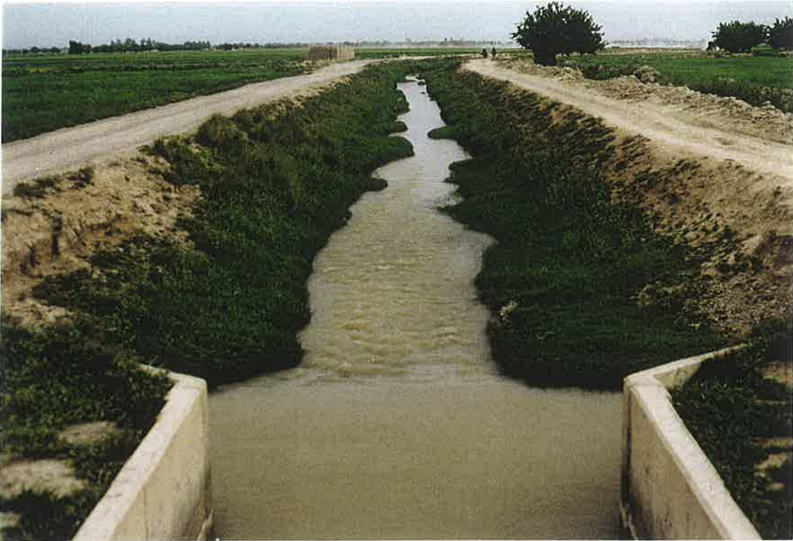
9. Silted banks of S-10.7 lateral at \pm Km. 29. 21 April 98
