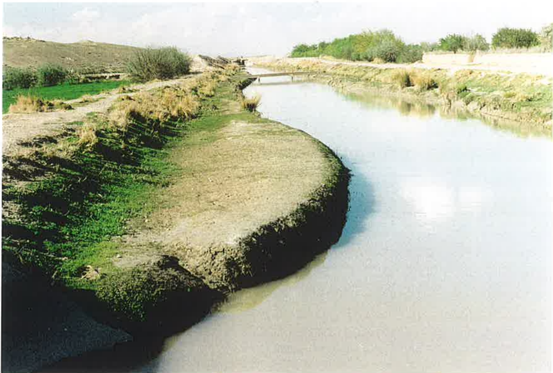
3. Silted Shamalan Canal at S-10.7 lateral intake (bottom left). This silt would be removed and used to fill the intake wing erosion in Photo #6. Water level is low. 21 March 1997.
