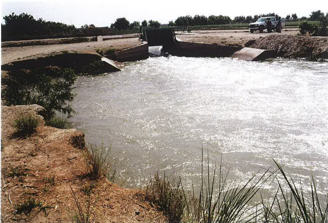
6. S-10.7 lateral intake gate off the Shamalan Canal with eroded wings and service road. 24 April 2000.
