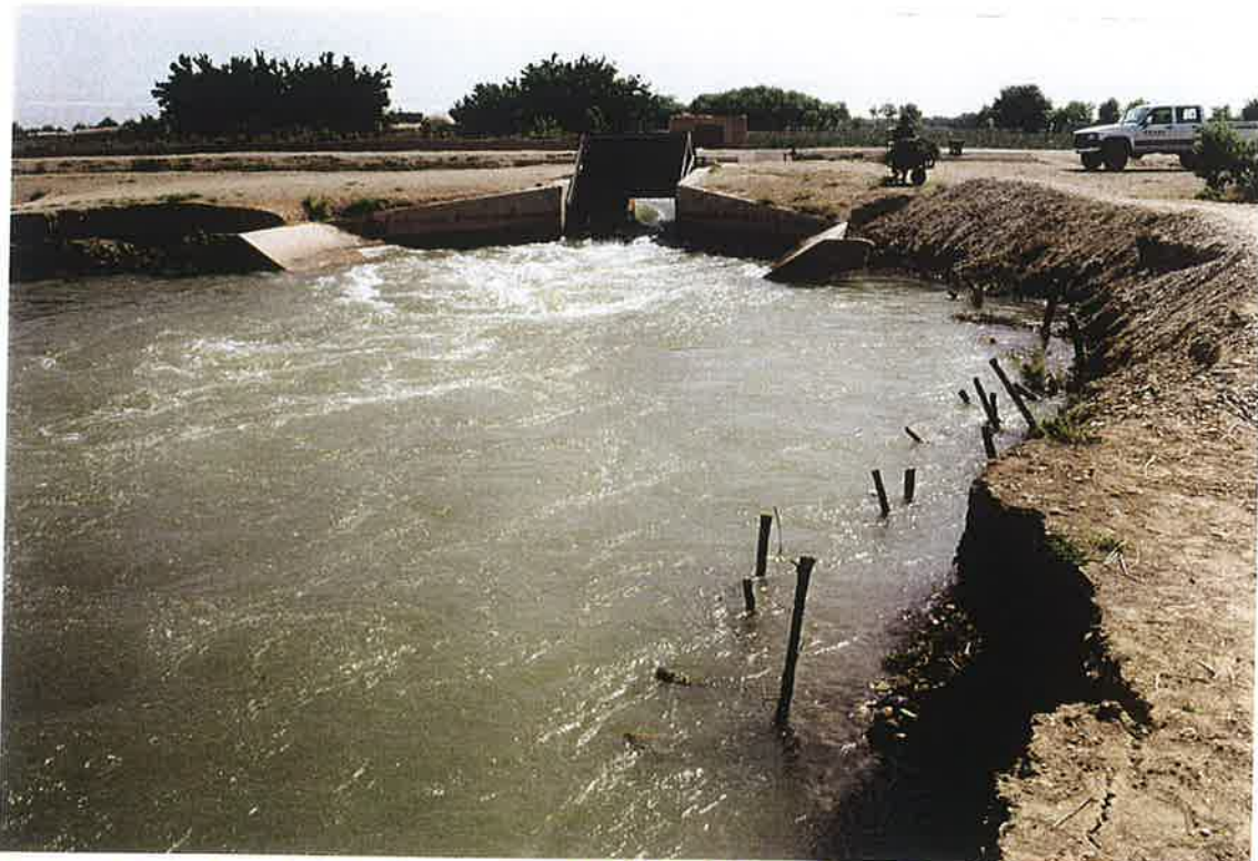
8. S-10.7 lateral intake gate off the Shamalan Canal with eroded wings and left bank service road. Note farmer placed sticks in an attempt at erosion control. The erosion resulted from years of no maintenance and the increase of water through the system. 24 April 2000
