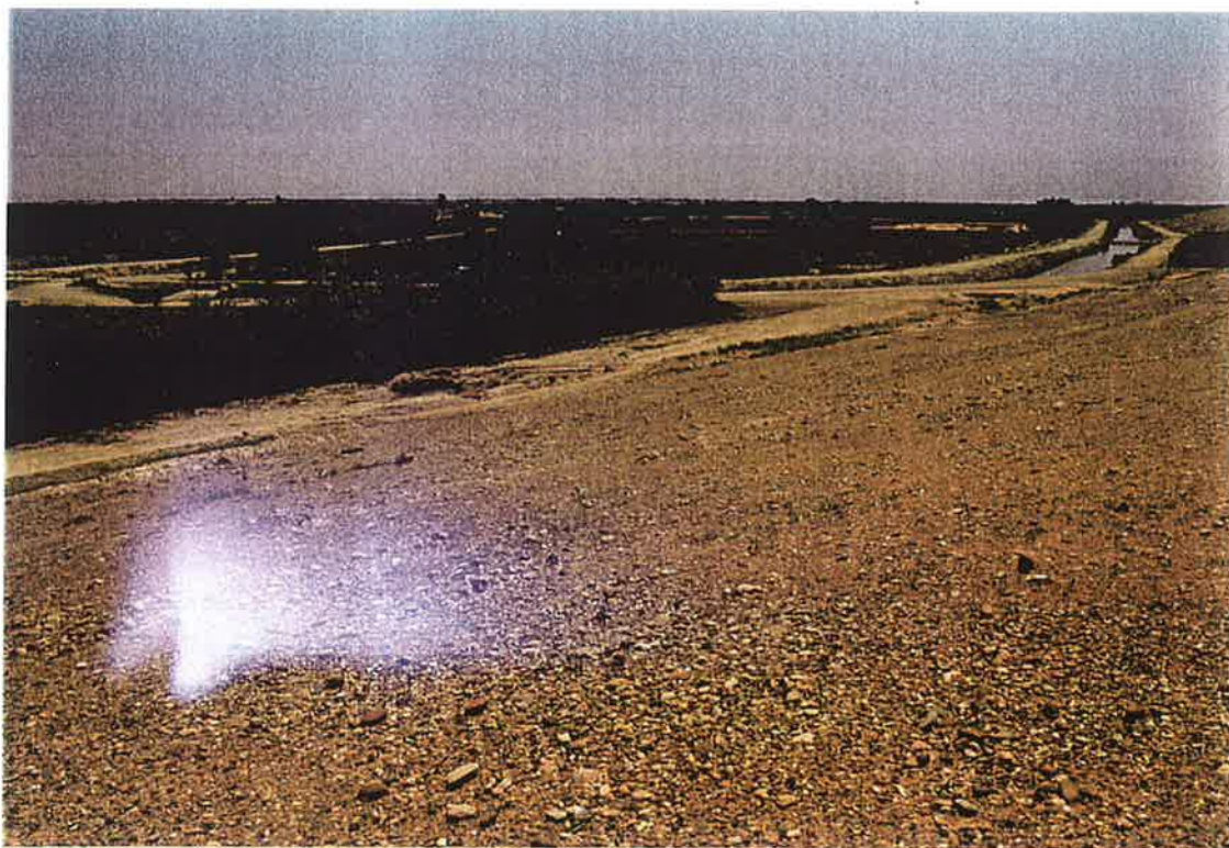
2. S-10.7 lateral at the Shamalan canal intake, Km. 0, on 20 April 1998. Note narrowing of channel by silt build-up.
