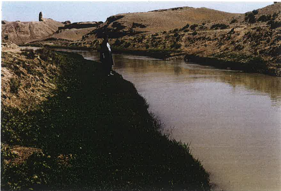
12. Silted banks of S-10,7 lateral at \pm km. 3. 20 April 98. HAFO Director, Engineer Jawed in center.
