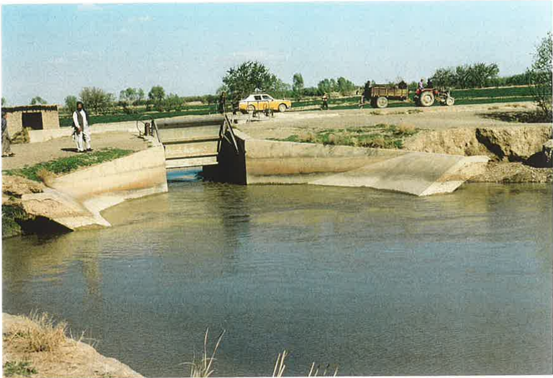
5. S-10.7 lateral intake gate off the Shamalan Canal. Note eroded wings and service road on right and left to be filled, compacted and stabilized with stone. HAKO Director, Engineer Jawed on left, 21 March 1997.
