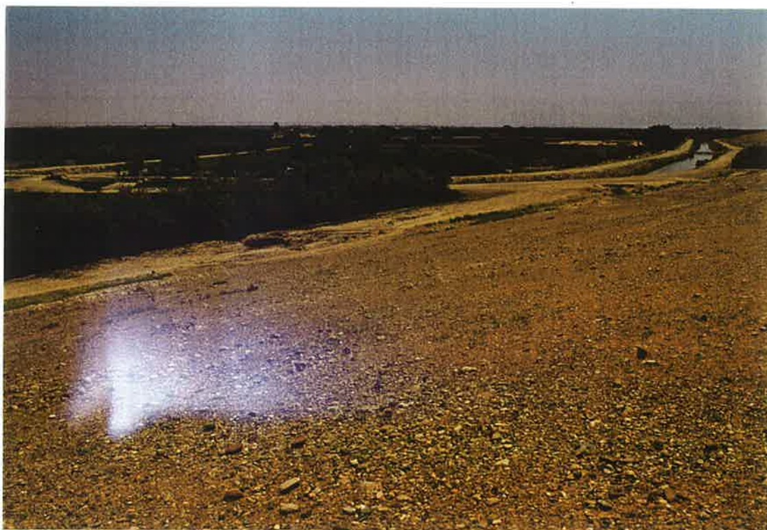
2. S-10.7 lateral at the Shamalan canal intake, Km. 0, on 20 April 1998. Note narrowing of channel by silt build-up.
