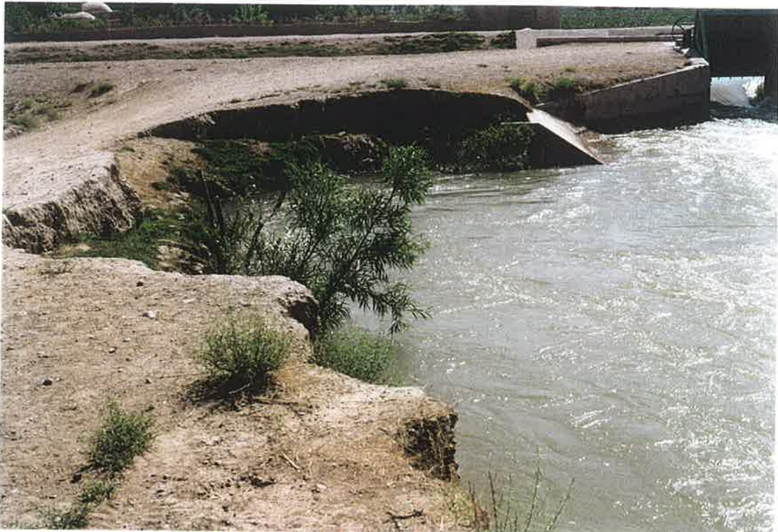
7. S-10.7 lateral intake gate off the Shamalan Canal (topright) with eroded wing and right bank service road. The sticks are placed by the farmers in hope that they will root and stop erosion. 24 April 2000
