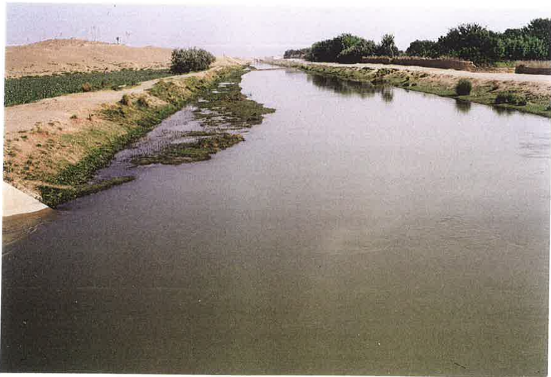
4. Silted Shamalan Canal at S-10.7 lateral intake (bottom left). Water level is high. 24 April 2000.
