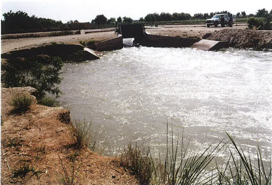
6. S-10.7 lateral intake gate off the Shamalan Canal with eroded wings and service road. 24 April 2000.
