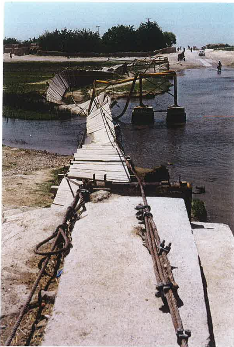
24 April 2000: Chan-I-Anjir footbridge from the west Chan-I-Anjir side. Note the vehicle ford top right.
