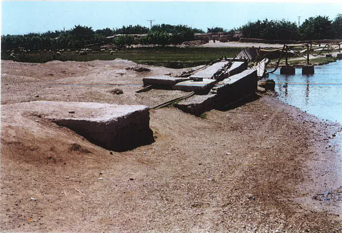
24 April 2000: Concrete approach to Chan-I-Anjir footbridge in need of repair, from the west. Note sizable village settlement across the wash.
