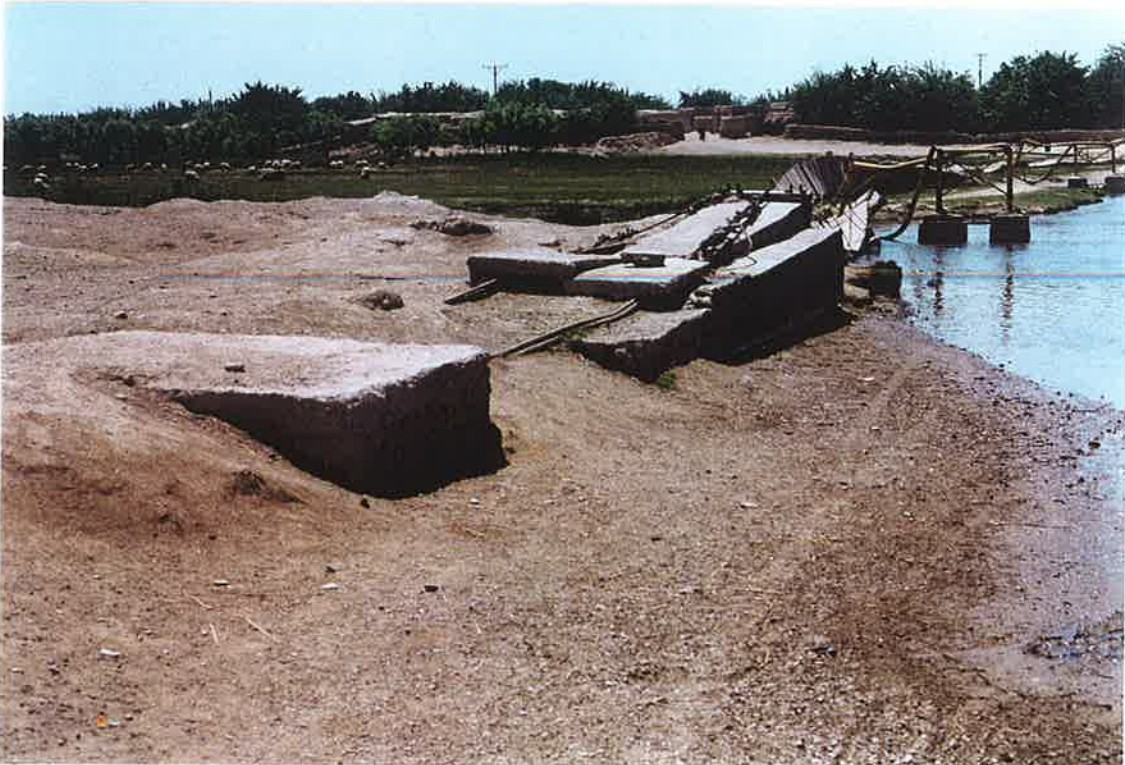
24 April 2000: Concrete approach to Chan-I-Anjir footbridge in need of repair, from the west. Note sizable village settlement across the wash.
