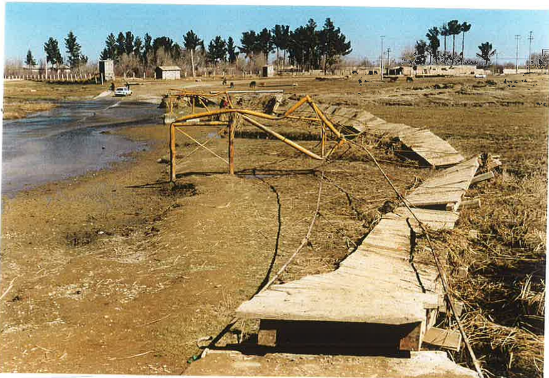
15 February 1999: Chan-I-Anjir footbridge in need of repair, from the east. Note vehicle ford on the left.
