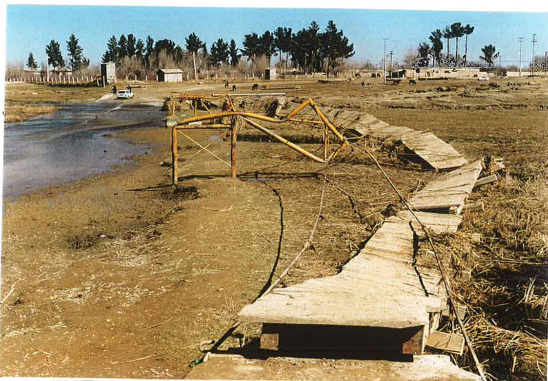
15 February 1999: Chan-I-Anjir footbridge in need of repair, from the east. Note vehicle ford on the left.
